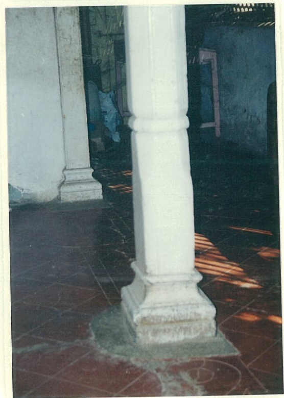
Carved timber column set in a carved stone base, in the front verandah
