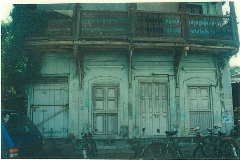
Projecting balcony supported on WI brackets. Lower floor kothars with timber frame structure
