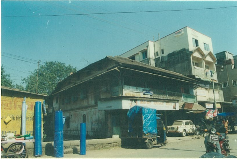
Corner view of the house showing overhanging roof at attic floor level and attic windows for roof ventilation
