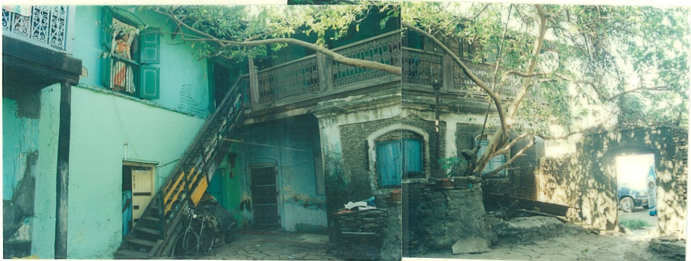
Panoramic view of the courtyard showing straight flight staircase leading to the upper floor corridor. Dindi Darwaza is seen on the right
