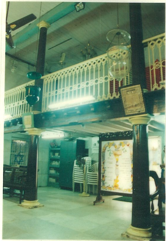
Mezzanine, supported on timber columns, articulated in the Tuscan manner, with ornamental cast iron grills
