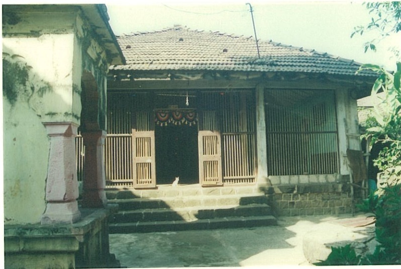
The open fronted temple in timber frame showing typically Konkan style construction and articulation
