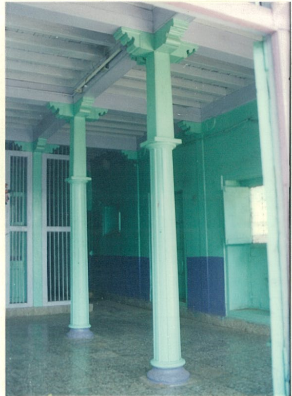
Carved timber column in the interior with carved brackets at the top and moulded stone base
