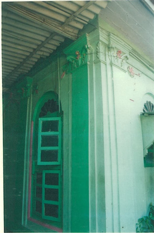
The corner view showing classically articulated pilasters, window bay and boarded eaves projection
