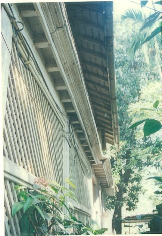
Front verandah with a slatted wooden screen protected by a deep overhang of the chhajja
