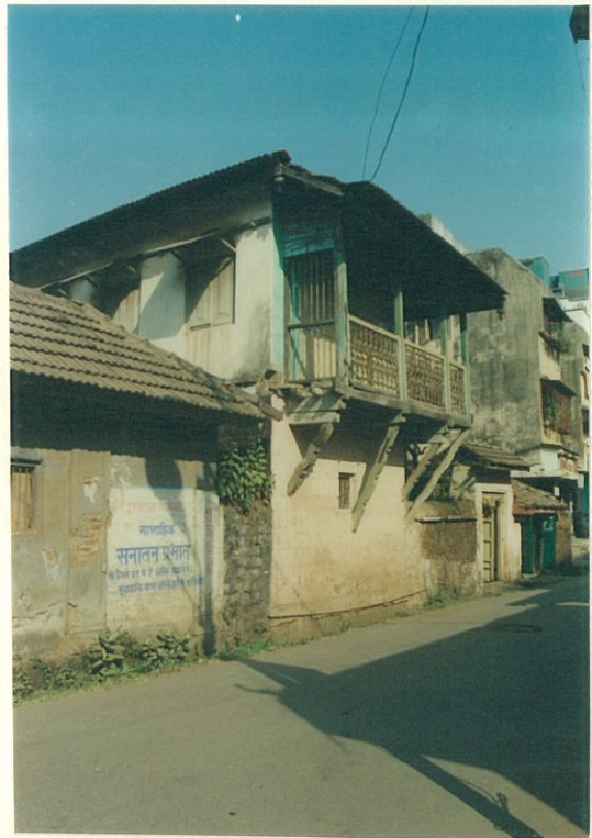
South corner view showing balcony projecting on the street and supported on TW brackets
