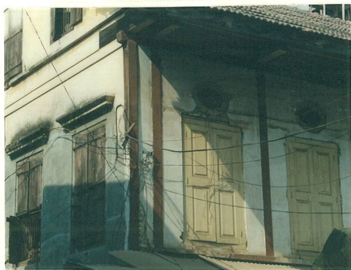
Corner view showing exposed timber frame Full height window with an oval fanlight
