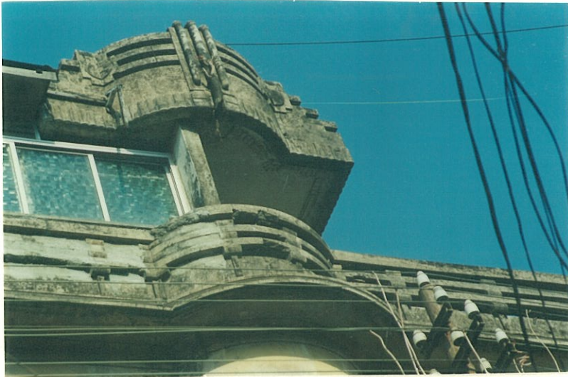
The protruding central bay with a culminating Art Deco motif at the top with three vertical strips
