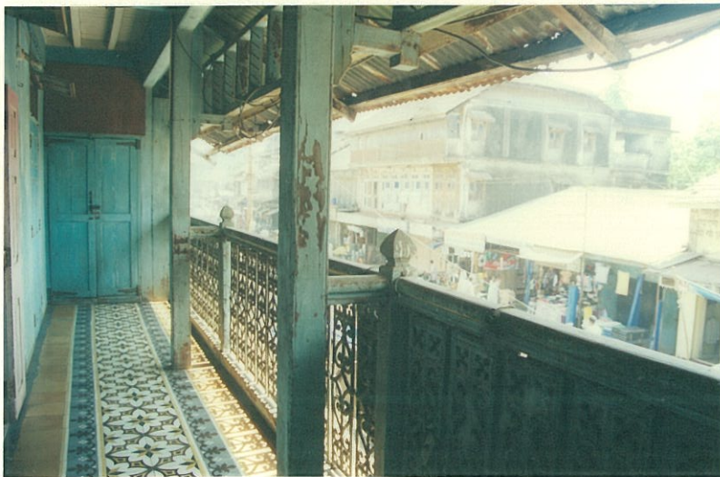
Upper floor balcony having a continuous balcony over the projected front. Also of note is floral floor pattern in coloured cement tiles
